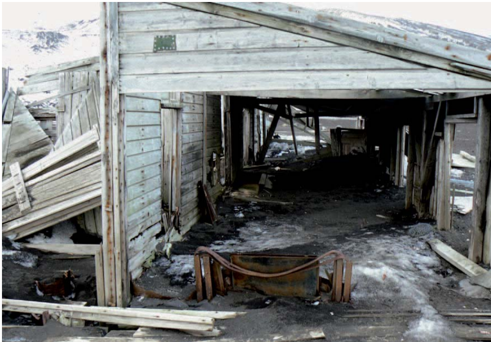
Figure 8. The dispensary/ store has been inundated with mud from a lahar. The mud holds moisture and microbes which creates a con- ducive environ- ment for decay to take place. Photo: Benjamin Held
