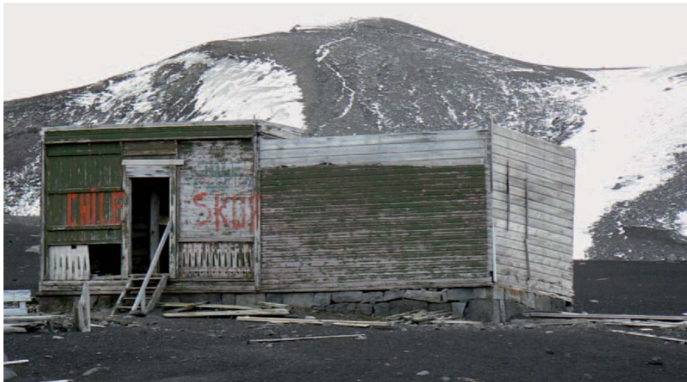
Figure 4. The Magistrate's residence has a solid foundation that has aided in avoiding deterioration by keeping the structure well above the soil. However, the roof has blown off exposing the interior to moisture. Photo: Benjamin Held
