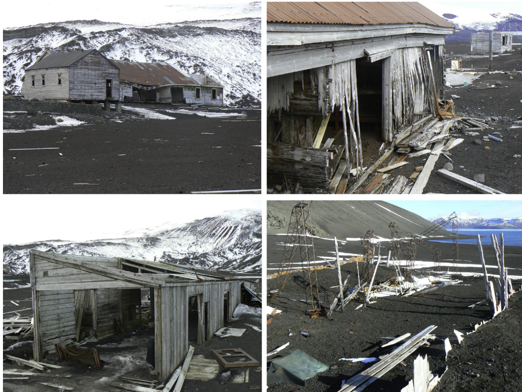
Fig 4 – The historic structures on Deception Island. Upper left; several structures showing buildings in various stages of decomposition. Upper right; the side of the Biscoe House, a building at Whalers Bay on Deception Island, showing extensive decay of wall boards and other timbers. Lower left; remnants of a structure that served as a dispensary/store that has been severely damaged by volcanic activity. Lower right; the remains of what was once the Chilean research base, Presidente Pedro Aguirre Cerda Station.
